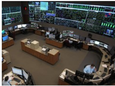
PJM's Valley Forge control room | NERC
